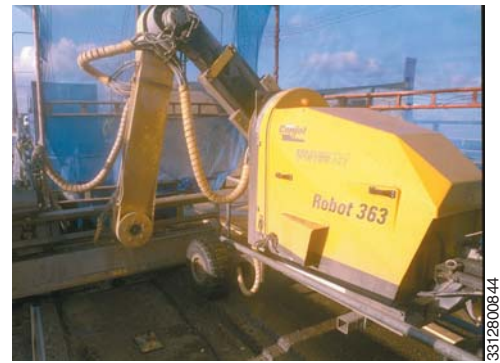
The Conjet Robot 363 removed per day in average some 30 to 35 m of deteriorated concrete from the edge of the deck.
