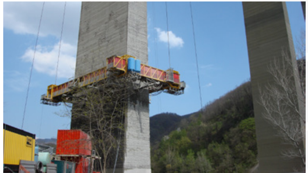
Repairs to the Rio Verde viaduct were performed from a special, purpose built cradle and working platform that wrapped round all four sides of the piers and supported by wire ropes connected to winches at ground level.
