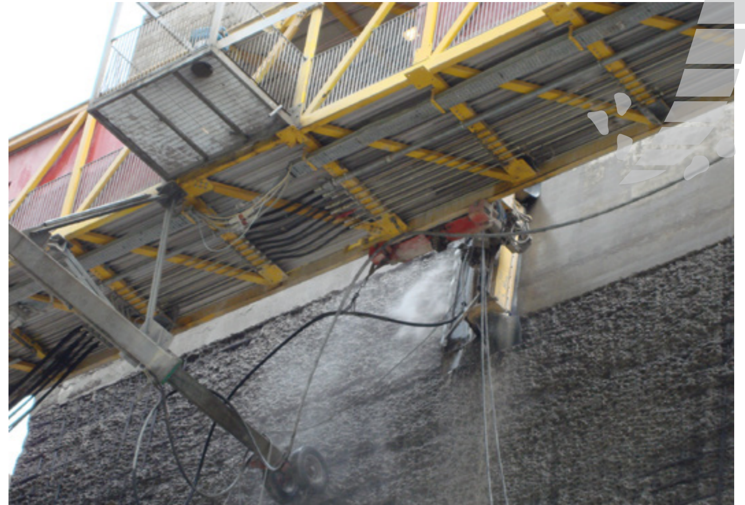
The Conjet modified feedbeam and nozzle, travelling back and forth along the platform's rack, selectively removed damaged concrete to a depth of 70mm and below any exposed reinforcement.
