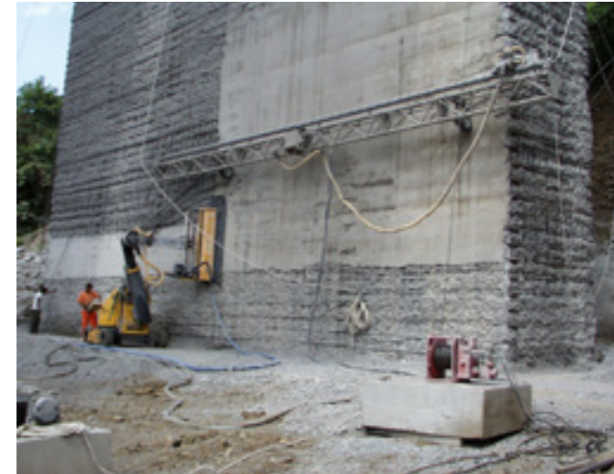
A Conjet Robot 365 at work on the bottom of a high-rise pillar.
