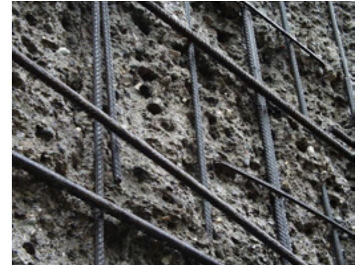
Exposed reinforcement, ready for the application of a new layer of concrete
