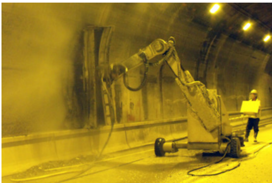
Conjet Robot 364 at work on the arched tunnel walls. The tool is specially adapted to fit the curvature of the wall for increased efficiency.
