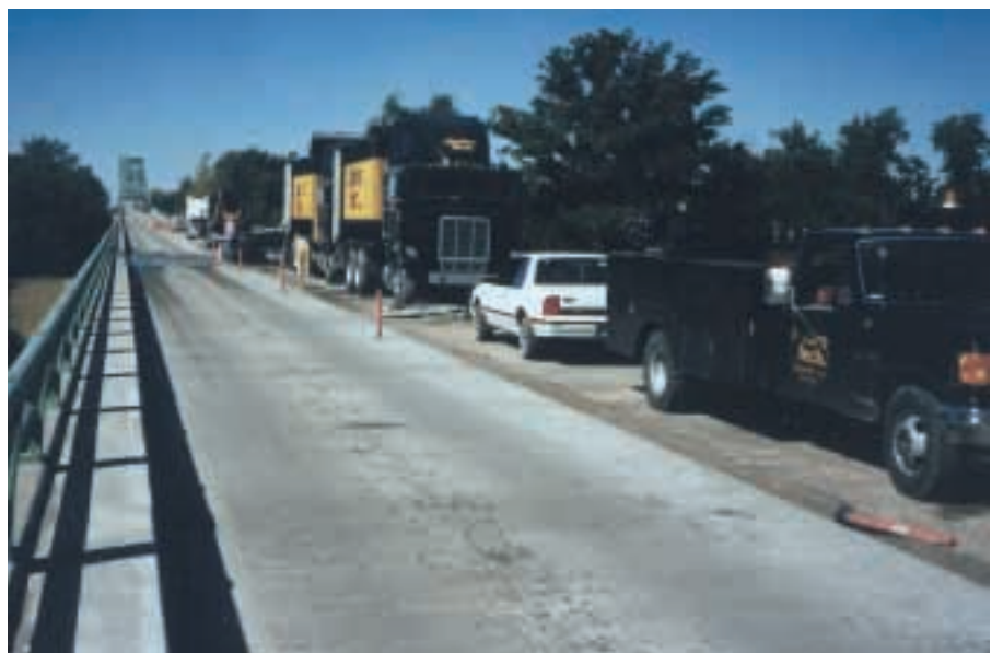
Below two Powerpacks and service truck parked along the 4,932 ft (1,480 m) long Wabash bridge.
