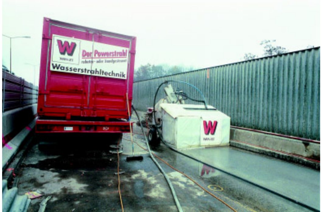
A Conjet 363 with an acoustic shroud made the concrete repair work at a bridge in central Zurich efficient and most of all environmentally friendly.
