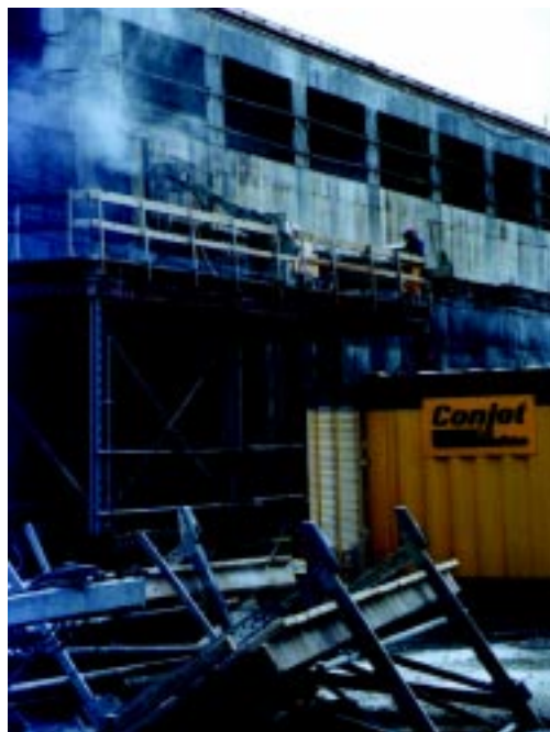
Contractor Belbetões is using its Conjet Robot 362 to selectively remove damaged concrete to a depth of 120 mm to 140 mm and below the reinforcement at an average rate of 1.5 m³/h.
