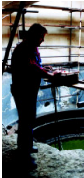
The operator monitors and controls the work progress, from a position above the working area.
