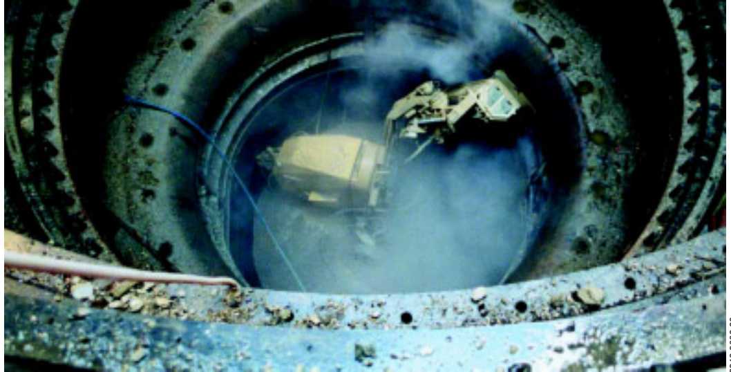
Conjet Robot 361 in the process of increasing the chamber diameter in the turbine draft tube.
