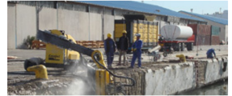
A Conjet Powerpack 345-360 kW supplying a Conjet Robot 364 MPA removing chloride damaged concrete from a quay. Clean water for the hydrodemolition process is supplied by the water tank trailer.
